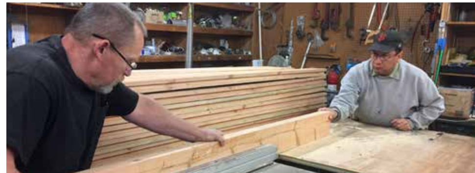
David Shell and Juan Villanueva take advantage of dry weather to prepare for deck repairs.
